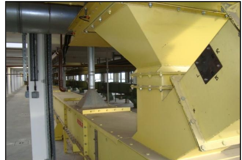
Boortmalt- Conveyor C111
