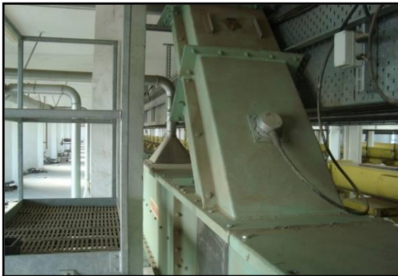
Boortmalt- Conveyor C103
